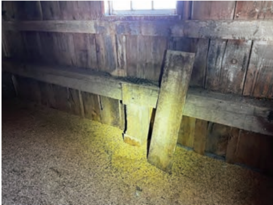
Photograph 2: Pile of bat droppings on upper level of granary.
