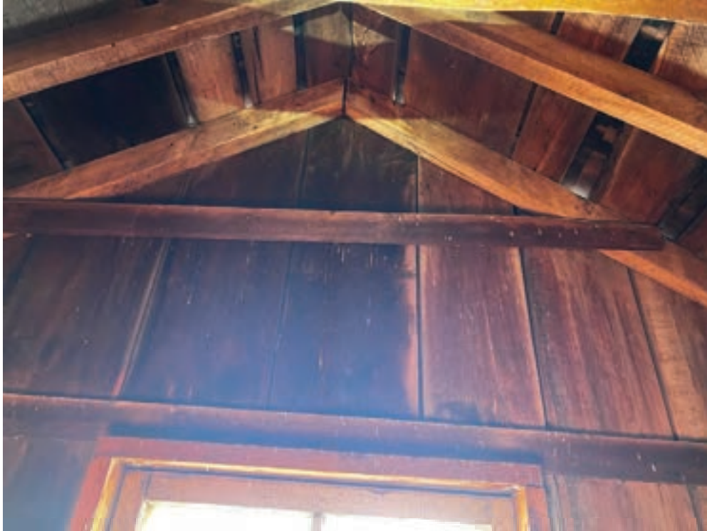
Photograph 3: Evidence of staining along rafters/walls of upper level of granary.
